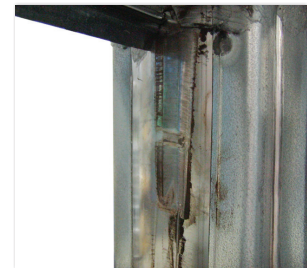
Appearance of damper seals after cycle testing
