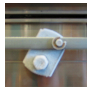
Close-up of frost build up linkage.
