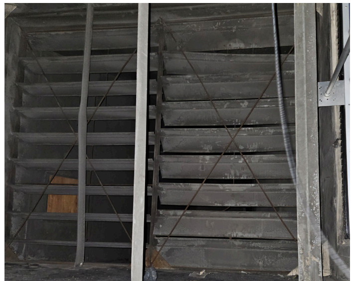
Fox Plaza's previous dampers were visibly inoperable - photo by Doug Miller
