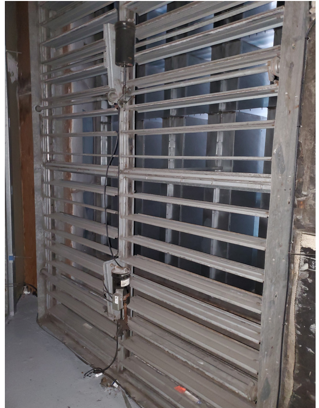
Galvanized steel rusts over time resulting in damper failure- photo by Doug Miller
