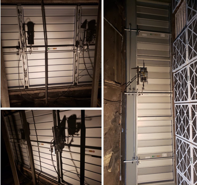
TAMCO Series 1000 Saltwater option dampers were installed throughout the Fox Plaza - photo by Doug Miller
